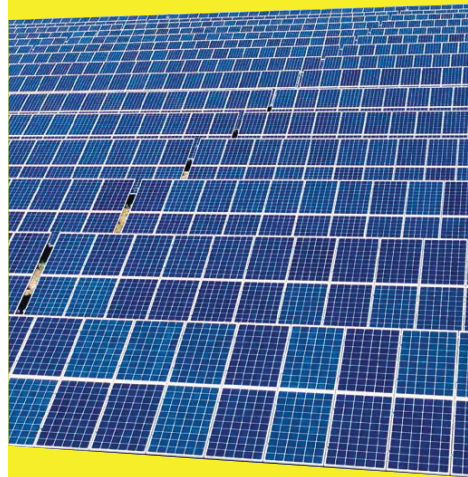
More than 700 kilometres (435 miles) of cable are installed at the photovoltaic farm in Braghin, Belarus.
